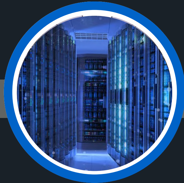
Advanced-Data Center Solutions
